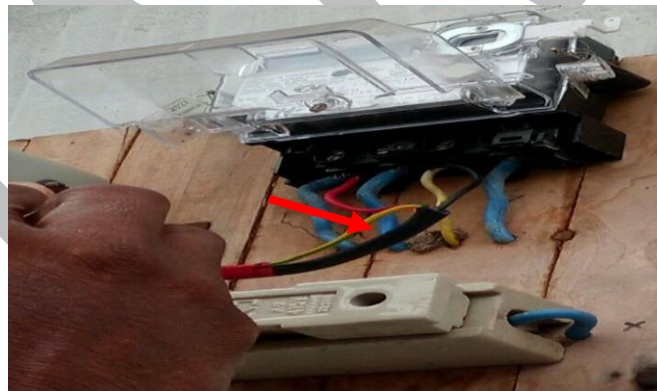
Fig.6. Direct Tapping In Single Phase Meter
